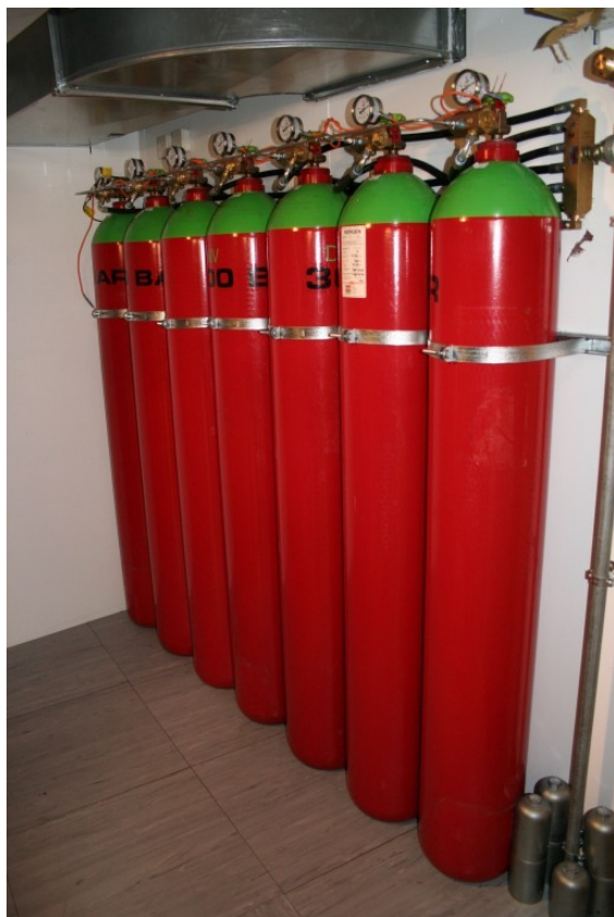
Cylinders containing argon gas for use in extinguishing fire without damaging server equipment
